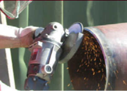
Edge chamfering a section of pipe with a Tiger Aluminum Back flap disc.
