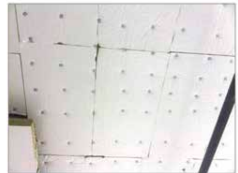
Over used stick pin installation. This increases the thermal bridge and reduces thermal efficiency.
