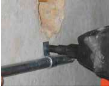
12HSMP034 clip assembly used to secure conduit
